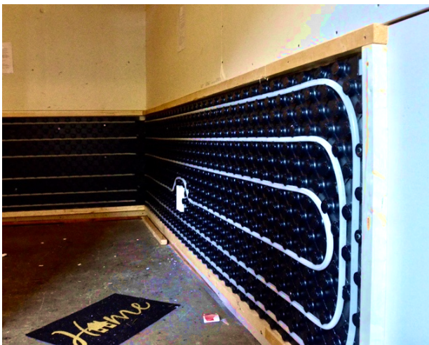
Heating tubes in the basement walls
